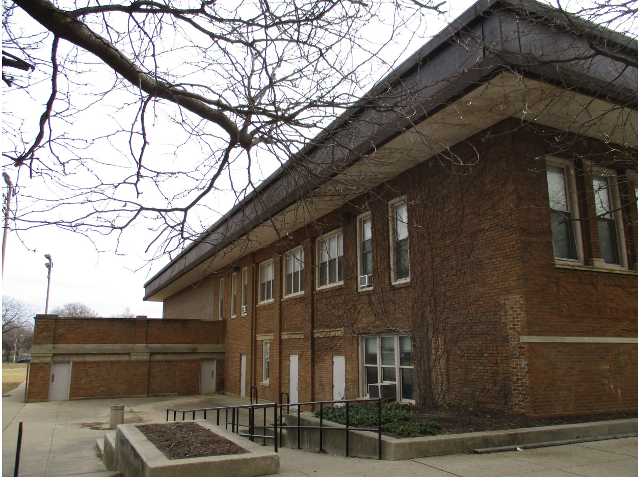
4501 N. Clarendon Avenue, view looking northwest from parking lot toward South façade
